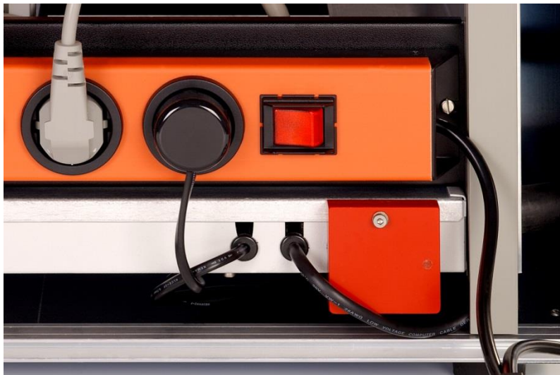
Figure 10: Switch of the distribution sockets on the back of the electronic device to switch on all electronic units.
