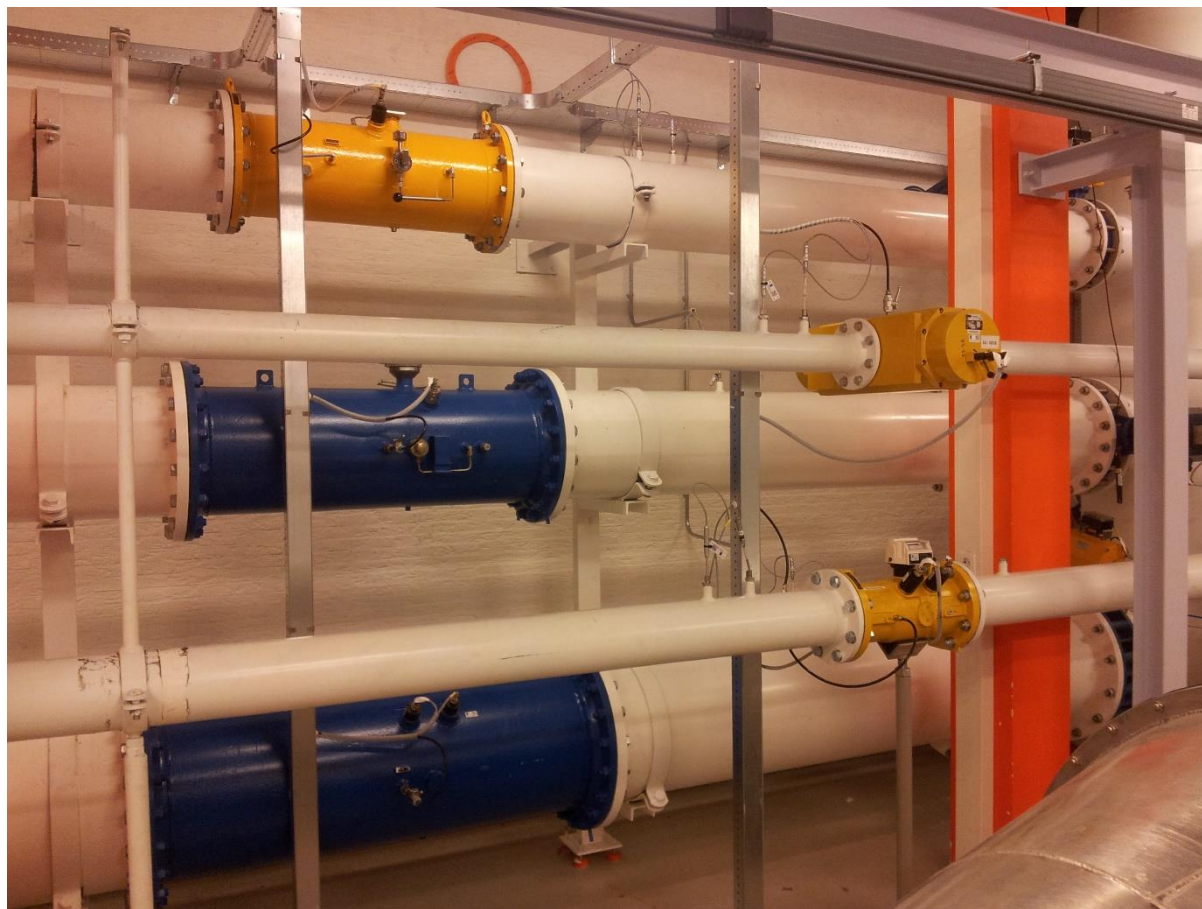
Figure 1 – The “Large Installation” facility at VSL with a range of flowrate from 15 to 15000 m 3 h -1 .
