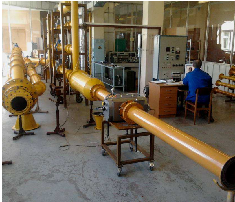
Figure 10 - The general view of the standard facility in Heat equipment research and testing laboratory of Lithuanian energy institute
